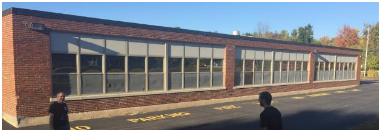
Poorly insulated walls, old windows and excessive window area, exposed slab edge make HPS expensive and inefficient to heat
